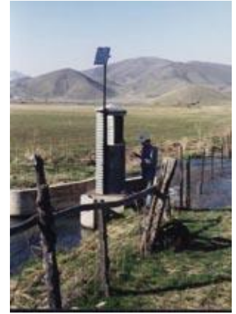
IEI personal performing annual calibration and maintenance
